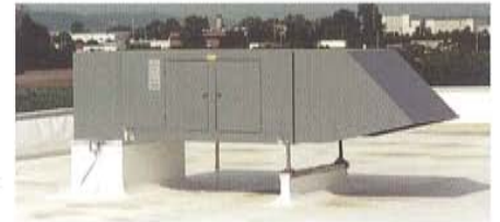
A typical Cambridge S-Series Blow-Thru Space Heater rooftop installation
